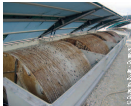
Rotating biological contactors
