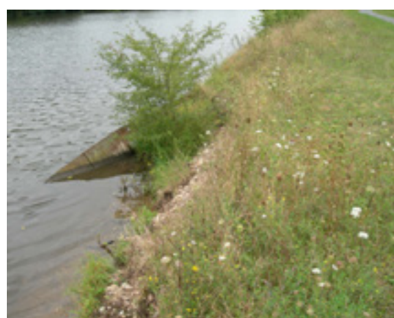
Collapse of sheet piles along 80 metres of the Moselle River. August 2008.
