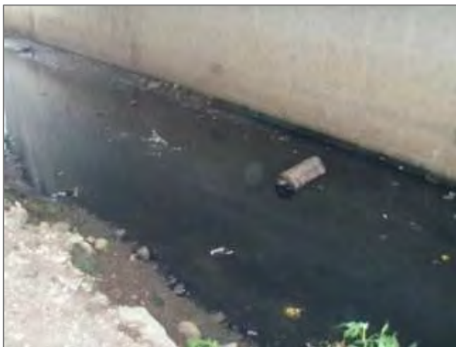
Stations d'épuration non conformes
